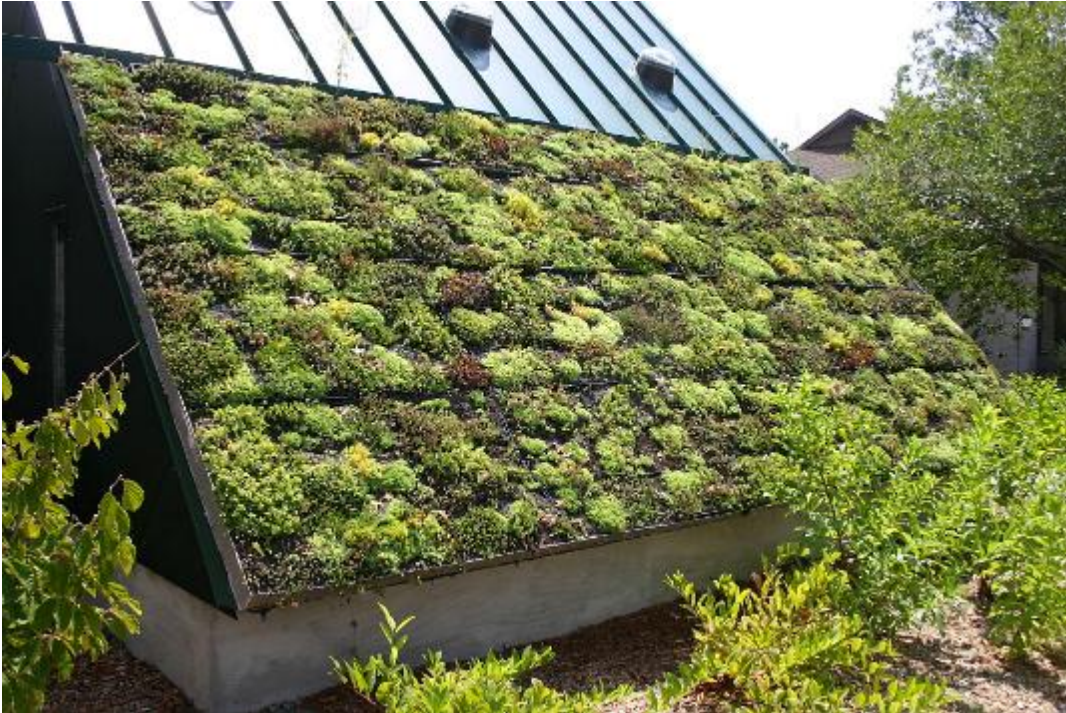
Eco-roofs manage stormwater with vegetated roof systems
